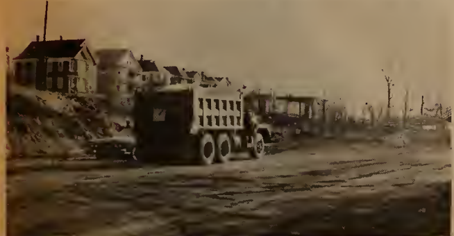
Spoils from the embankment excavation are hauled away in heavy dump trucks. The dirt is covered with canvas to prevent spillage onto city streets.
